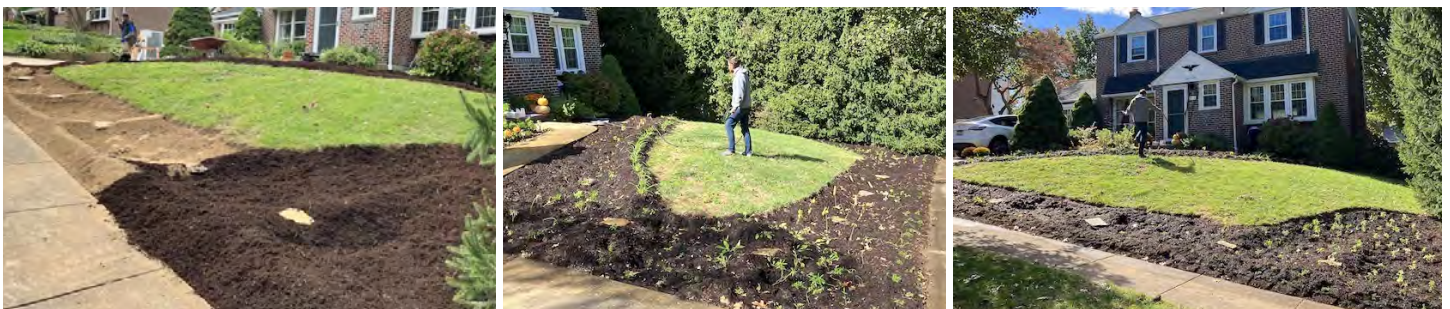
Residential Rain Garden during Installation- an appropriate site is selected, prepared, and then planted
